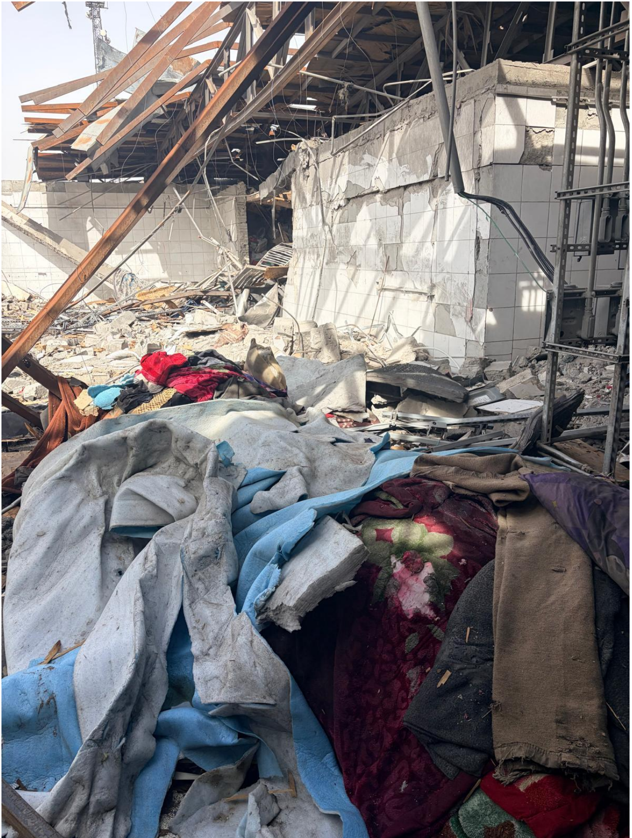
Image of damaged sleeping quarters, Omid Rehabilitation Hospital, 24 March 2026
