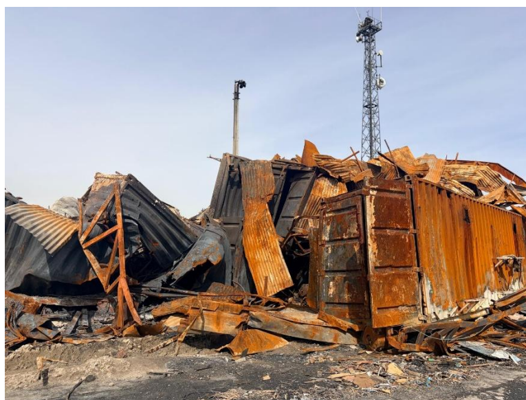
Image of damaged structures, Omid Rehabilitation Hospital, 24 March 2026
