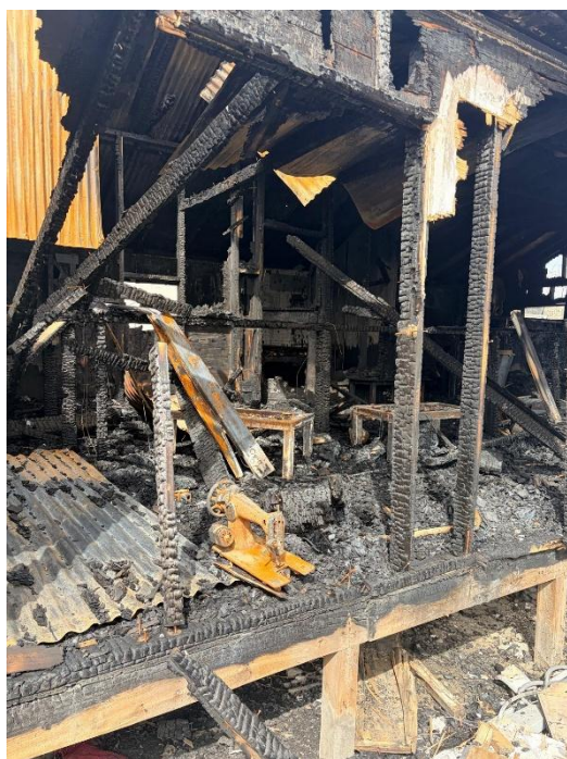
Image of damaged vocational training area, Omid Rehabilitation Hospital, 24 March 2026
